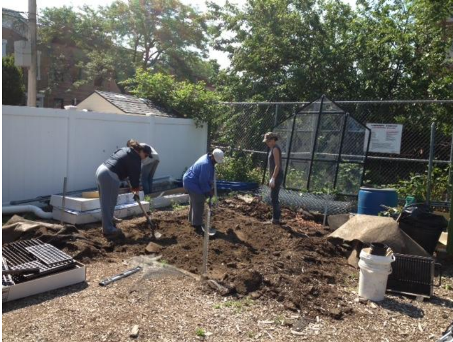
Community members prepare the foundation for the greenhouse at the People's Garden.
